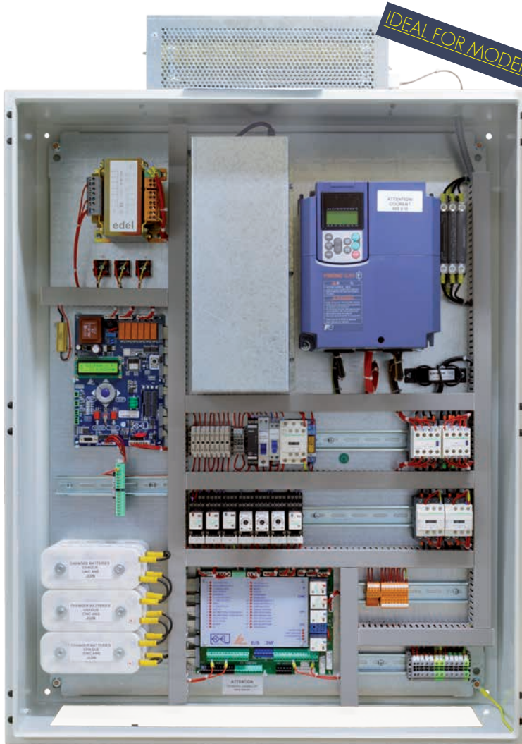
Controllers with rescue unit powering the motor, with door opening on reaching the landing.
