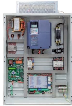
K2 controller cabinet
