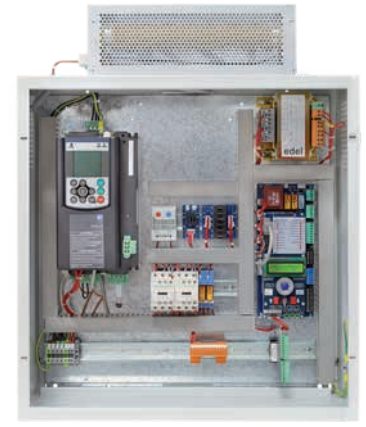
Advanced K2 controller cabinet
